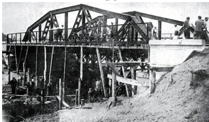
Fig. 3. Wooden scaffolding under the span of the bridge over the Słudwia river in Maurzyce [13]
