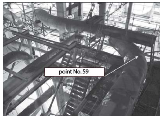
Figure 19. One of points of measurement by AE of operation activity of pipeline of steam intermediate overheating at Kiev HES-6
