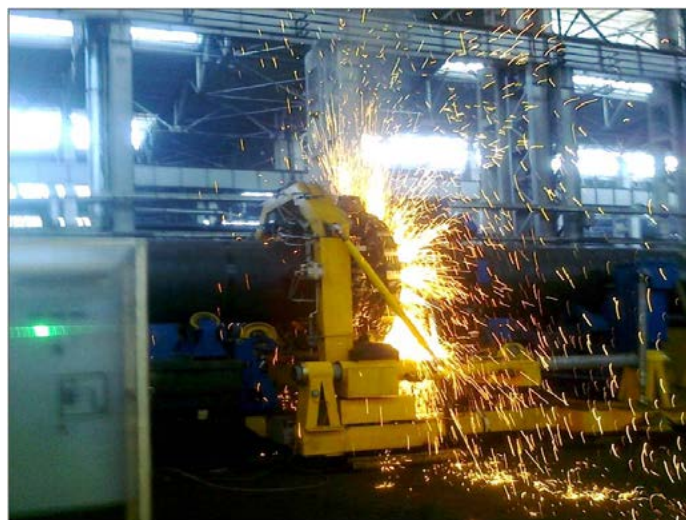
Figure 16. Equipment for flash-butt welding of offshore pipelines of 1219 mm diameter and 27 mm wall thickness
