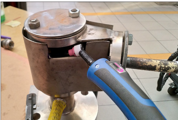
Fig. 19. Device used during the repair welding of the injector tube (during assembly)
