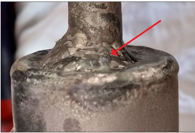
Fig. 18. Weld with the crack
