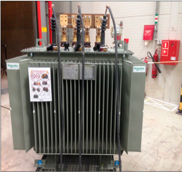
Fig. 2. Measurement points 1–5 marked on the radiator of the 1600 kVA transformer
