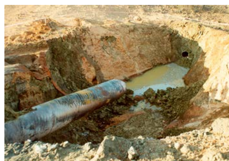
Fig. 9 Situation after explosion
