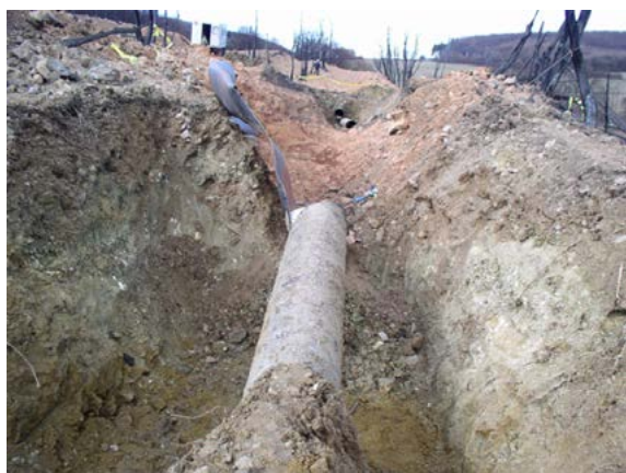
Fig. 7 Breakdown of the 1 st international gas pipeline (OD 720 mm)
