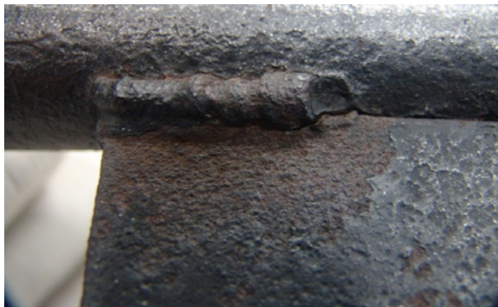
Fig. 13. Crack (partly torn weld) on the length of 15 mm in weld on upper left side of letter "E" in word FREI
