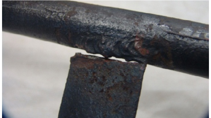
Fig. 15. Weld joining the letter "I" with upper pipe in word FREI – letter broken off on the whole length of welded joint (part of weld remained on pipe)
