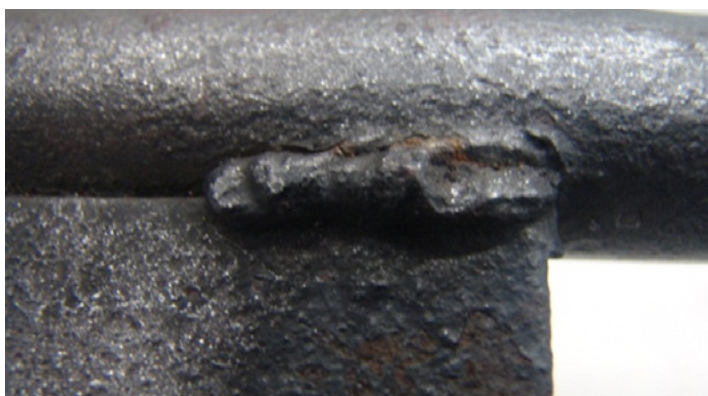
Fig. 14. Weld torn off, located on the upper right side of the letter "E" in word FREI (weld torn of on the length of 37.5 mm)
