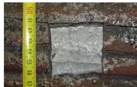
Fig. 10. Torn-off fragment of the high-chromium cast iron-surfaced layer
