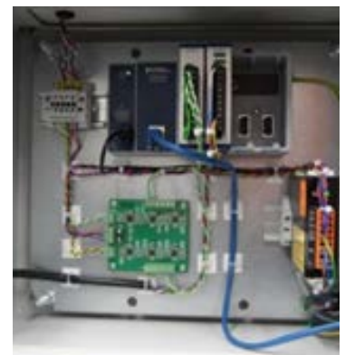
d) inside the measurement module
