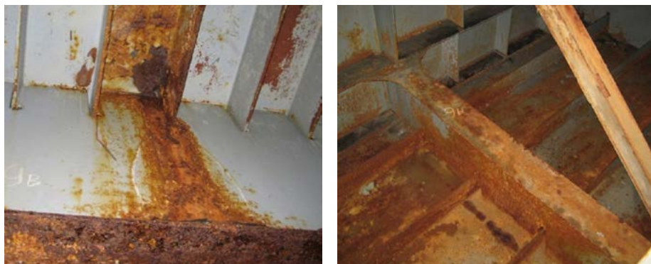
Fig. 1. Corrosion damage to the main beam of the box section of a road bridge
