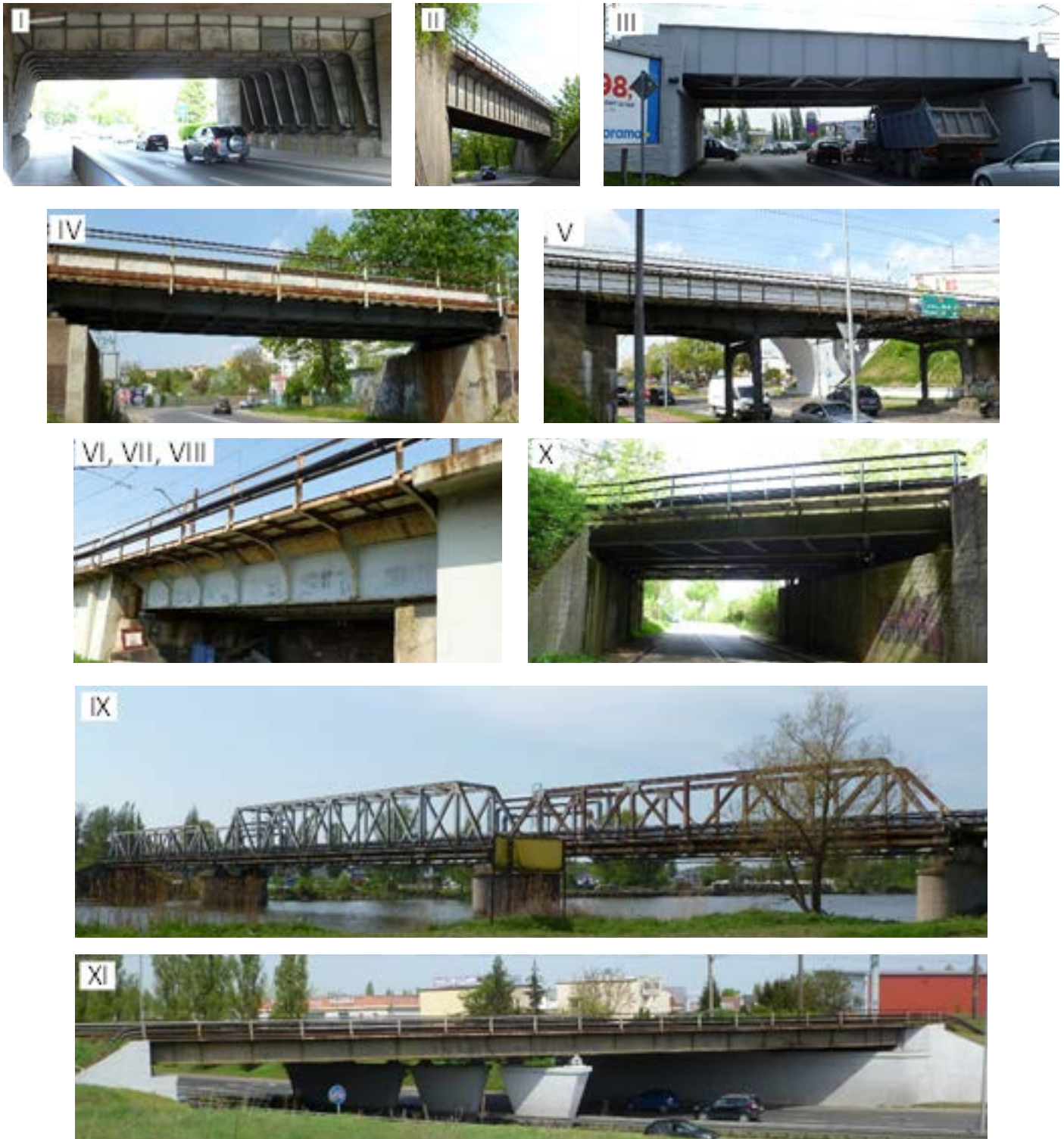
Fig. 3. Bridges subjected to the tests (bridge no. VI, VII and VIII of the identical structure)
