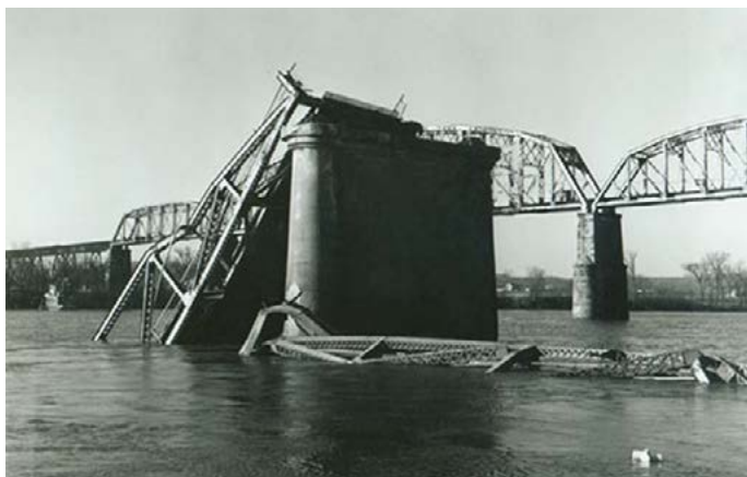
Fig. 3. Bridge collapsed due to corrosion and stresses in Point Pleasant in 1967 in the USA
