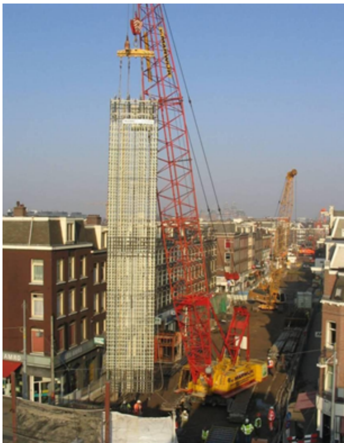
Fig. 7. Reinforcement of the soft-eye wall made using composite rebars (21 metres in height) [18]
