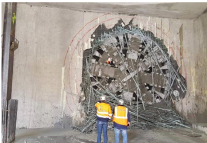
Fig. 8. Penetration of a soft-eye wall by the Maria boring shield; construction of the north-east section of Warsaw underground line II [19]
