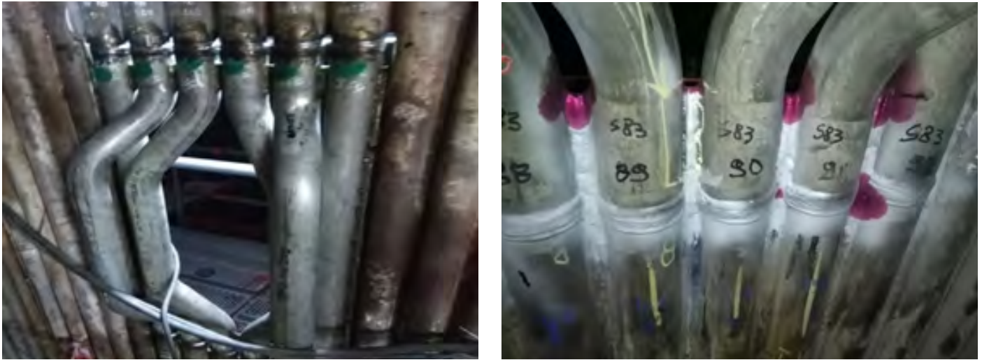
Fig. 1. Use of composite tubes: a) deflection for the nozzle in the combustion chamber (made of tubes 3R12/4L7) and b) waterwall of the soda recovery boiler (made of composite tubes)
