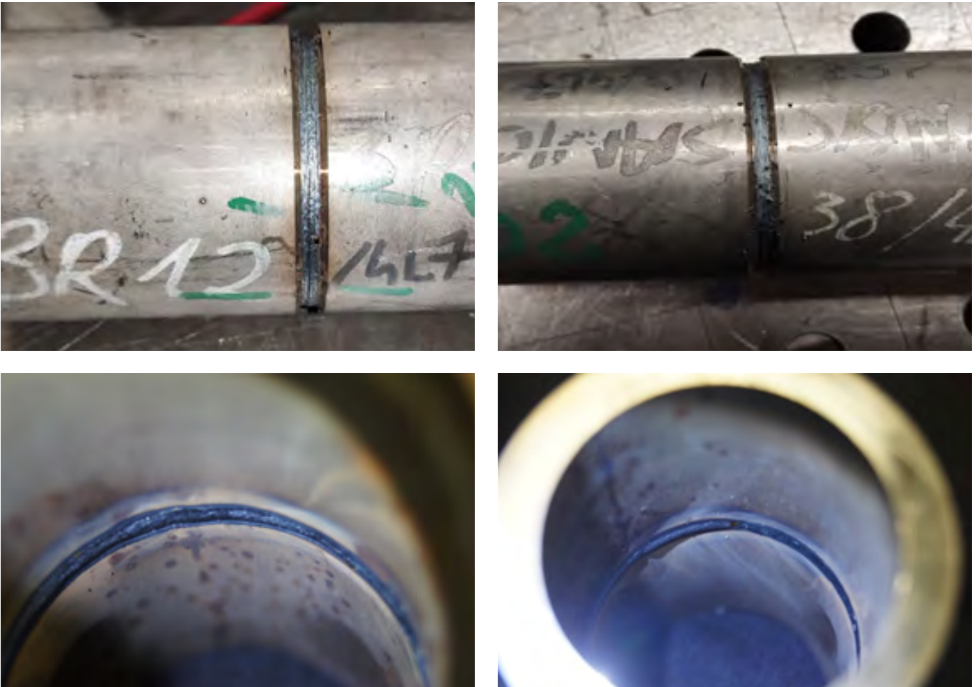
Fig. 7. Laser joint of the internal layer viewed from the weld face and weld root side: a) weld face and root – tube grade 3R12/4L7 and b) weld face and root – tube grade Sanicro 38/4L7
